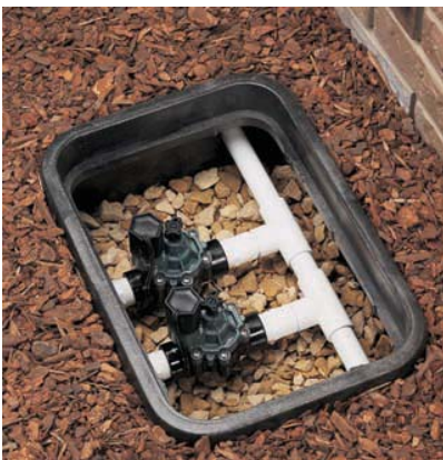
Two valves in a valve box. ©2006 Rain Bird Corp.
